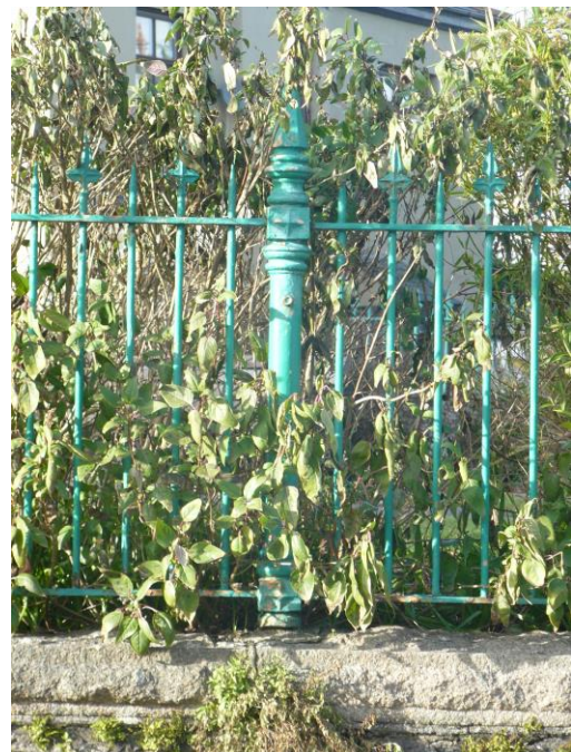
corroded newel post on southern boundary
