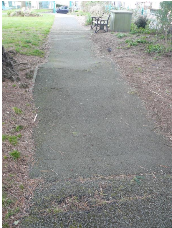
displaced tarmac adjacent to fir tree
