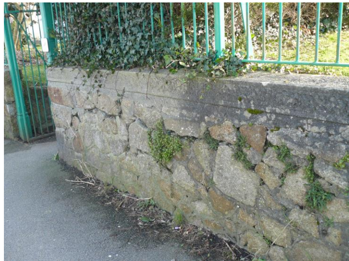
example of weed growth & defective pointing
