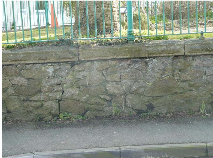
displaced masonry adjacent to Araucaria Araucana tree
