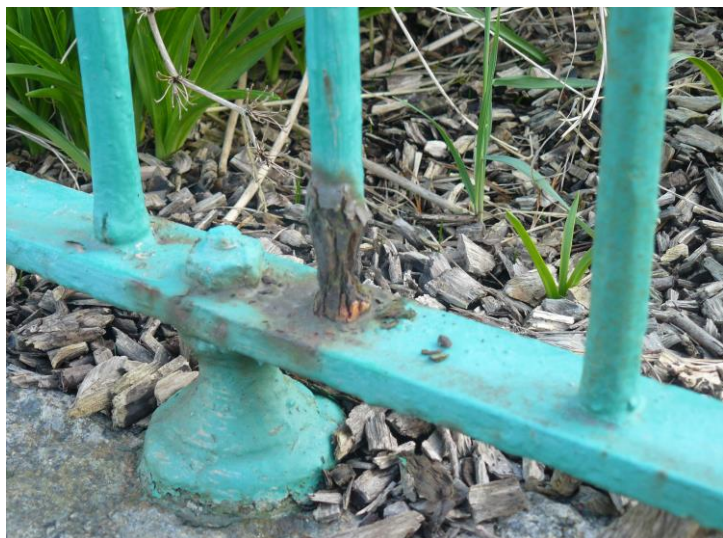
example of corrosion to metal railings
